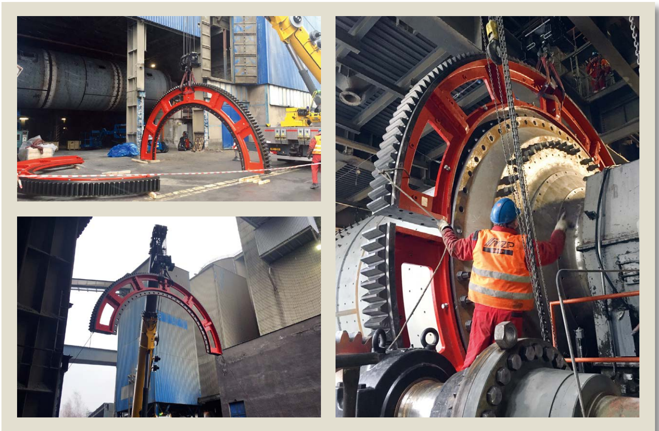
Figure 3: Because the segments can be pre-assembled in two halves, handling on site is considerably simplified (Photo: Cemex)
